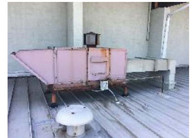
Society Bldg Make-Up-Air Unit
