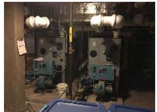
Society Bldg Boilers
