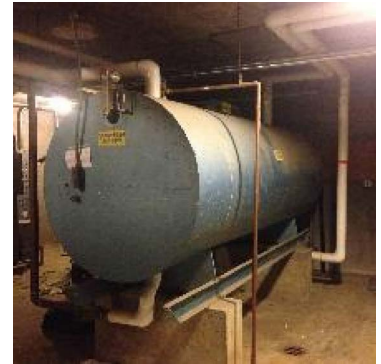
Society Bldg Hot Water Tank
