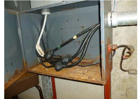
Primary Bldg Splice Box
