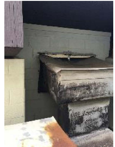
Society Bldg Damaged Ductwork
